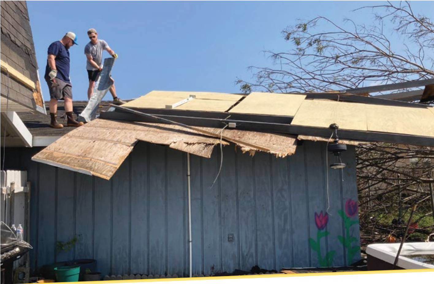
Danos Employee work together to help the community with Hurricana Ida cleanup and repair efforts.
